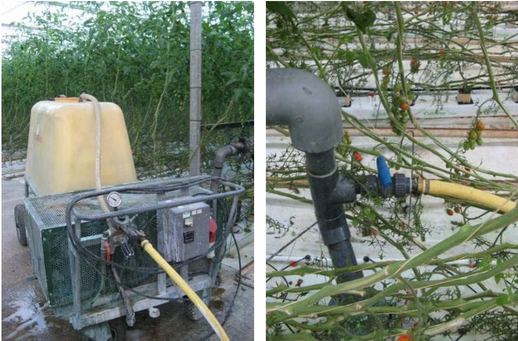
Figure 17. Showing (left to right) the spray tank / pump and the attachment to the irrigation manifold.
